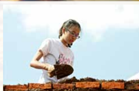
Shinhee Kang, grade 10, pitches in with the construction effort on the new school.
